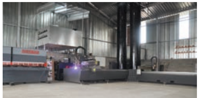
▲ A fully equipped fitter and turner shop serves the workshop with parts and all bending and cutting are done in-house.
